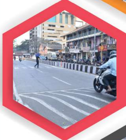
Construction of Speed Breaker as Speed Calming Measures In Front of School
